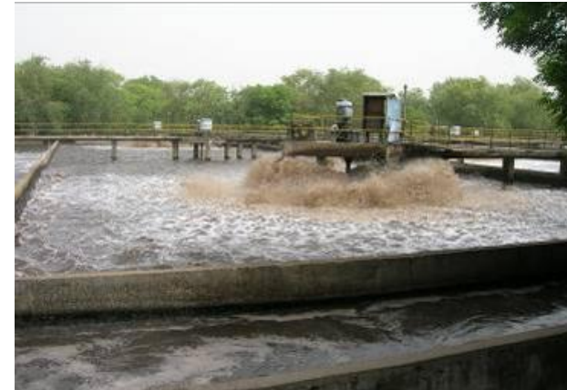
Dilapidated sewerage treatment facilities
